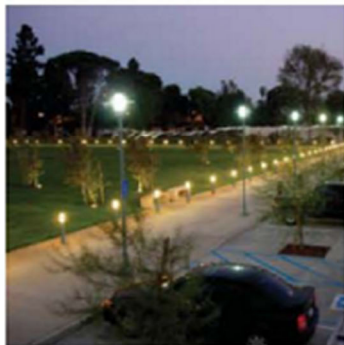
Pedestrian overhead + bollard lighting
