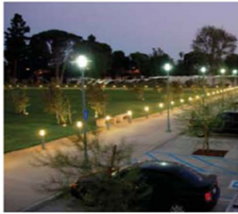
Dark-sky pedestrian + bollard lighting
