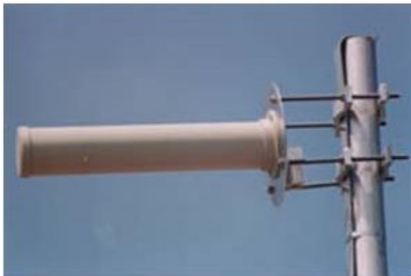
Exhibit 9. The antenna extends horizontally from the pole. This design is prohibited.
