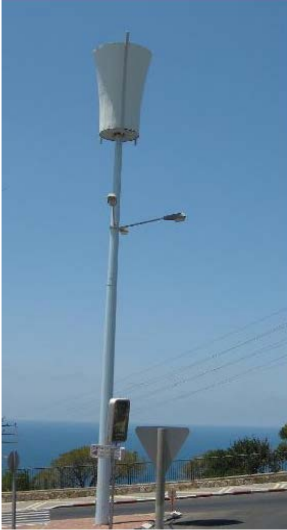
Exhibit 8. The antenna is wider than, and out-of-scale to the pole. This design is prohibited.
