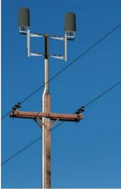
Exhibit 6. Wireless facilities over, or within 20 feet of energized wires are prohibited.
