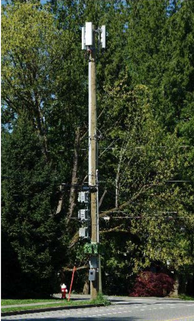
Exhibit 10. Wooden poles are prohibited. In addition, t The top-mounted antennas extend on arms away from the pole. This design is prohibited.
